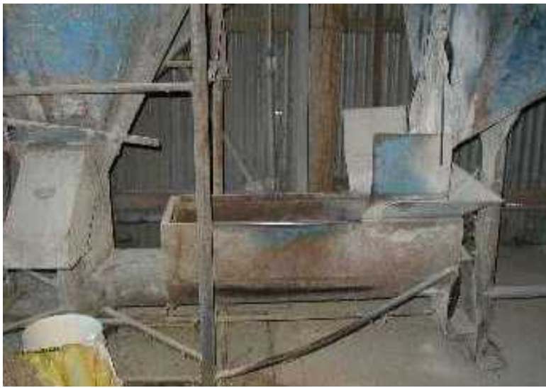
Figure 3.5: Animal feed mixing plant
