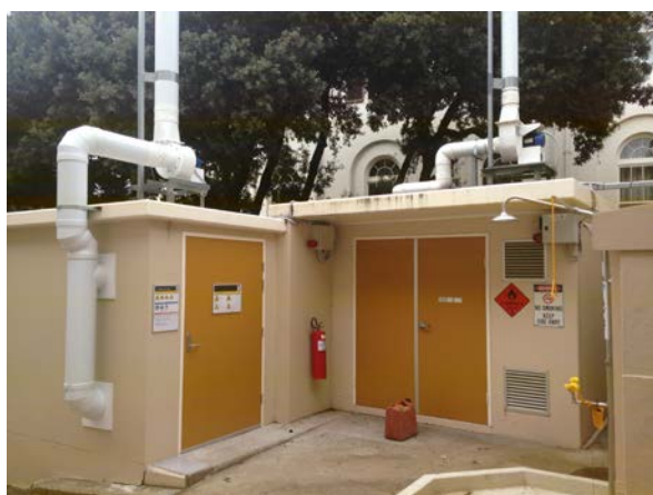
Figure 5: Class 3 flammable liquids Dangerous Goods depot
