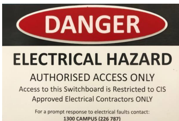
Image 3 – Example of Plant Room Sign
