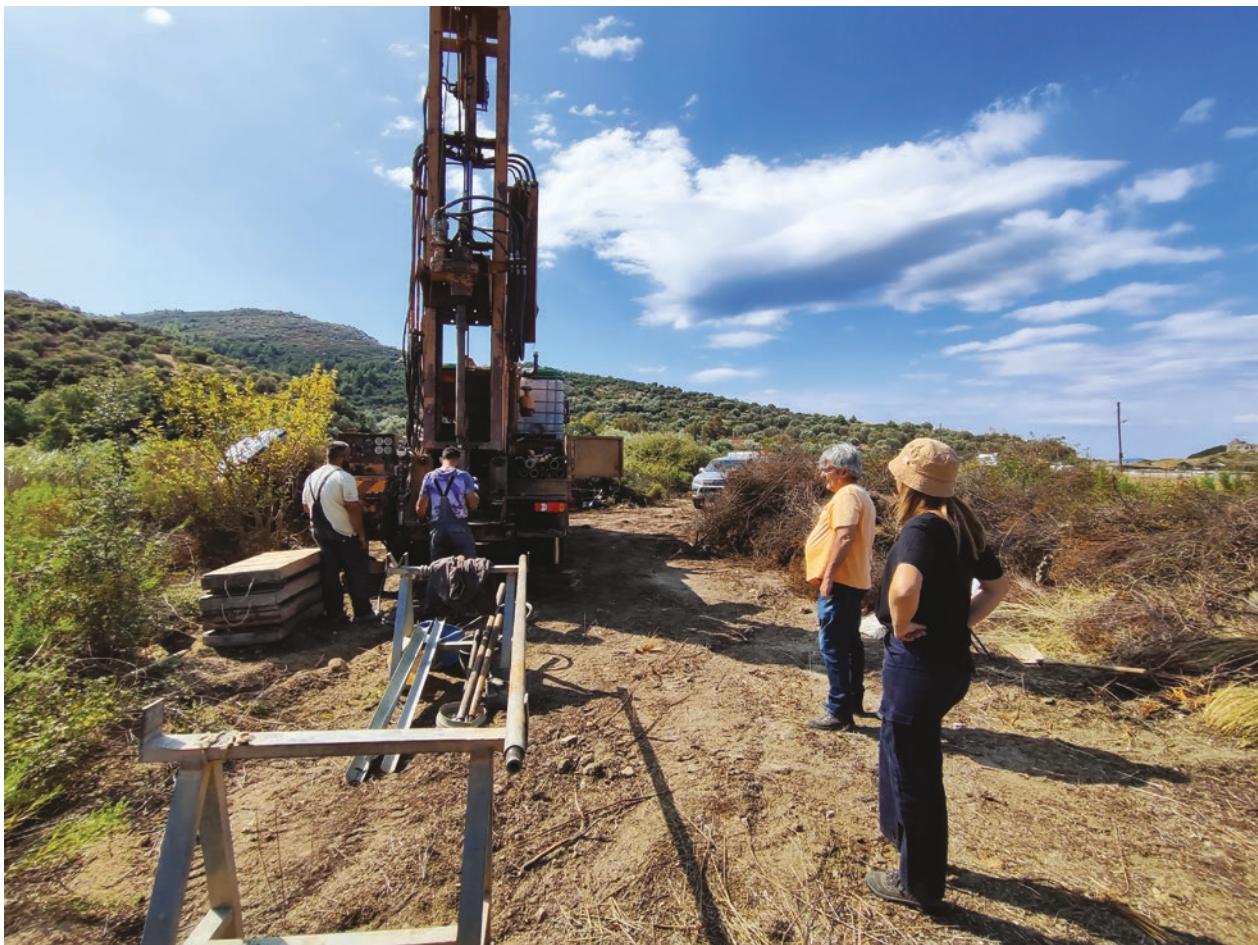
Fig. 5. Drilling commences, 18 September 2023 (the peninsula known as the Lekythos can be seen on the distant right)
