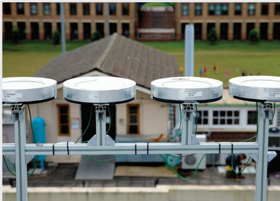
Dewpoint Innovations technology on the Sydney Nanoscience Hub rooftop as part of Sydney Nano Living Lab pilot program
