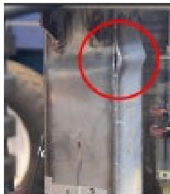
Local buckling and weld fracture
